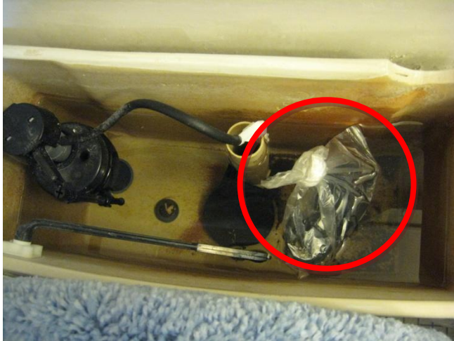
Figure 2: Photo of temperature sensor in toilet tank
